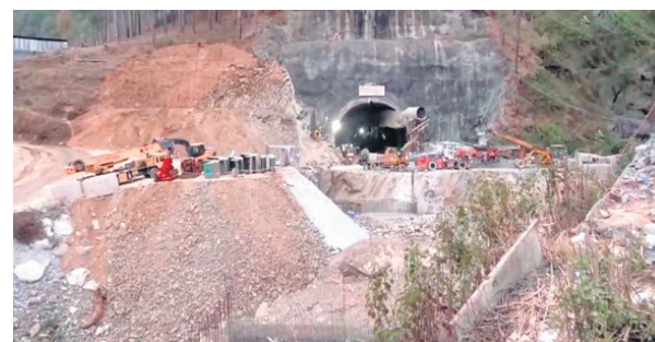
Rescue operation is underway in the Silkyara tunnel where 41 workers are trapped inside after a portion of it collapsed, in Uttarakhand on Monday. ANI
