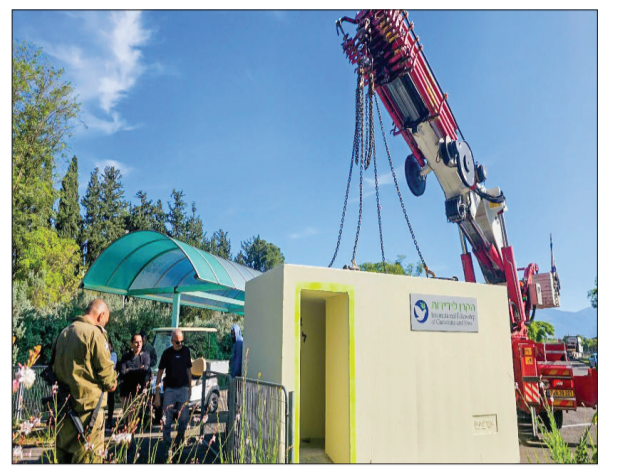
One of the mobile bomb shelters to be installed.
