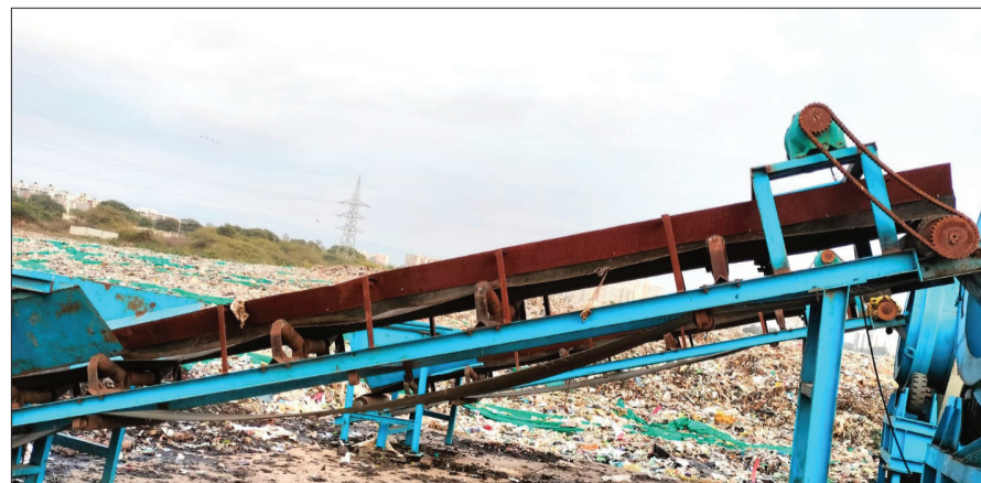
View of two of the trommel machines getting damaged due to rain water
