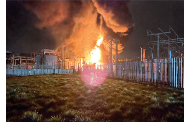
A massive power outage, triggered by a fire at a nearby electricity substation in London. Agency
